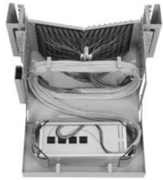
Top Cover Removed (splicing area open)
